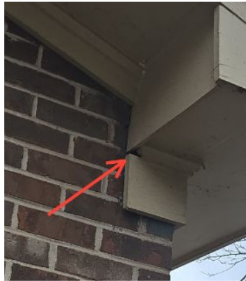
Open access to attic for pests.
