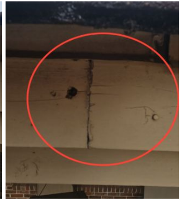
Exposed nail and wood. Seam needs to be sealed
