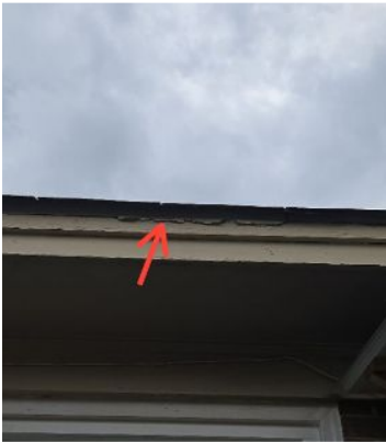
Paint lifted from wood surface from drip edge movement.
