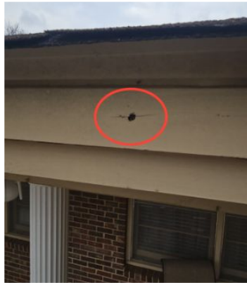
Exposed nail and wood
