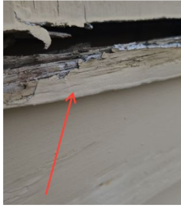
Close-up of rotten wood
